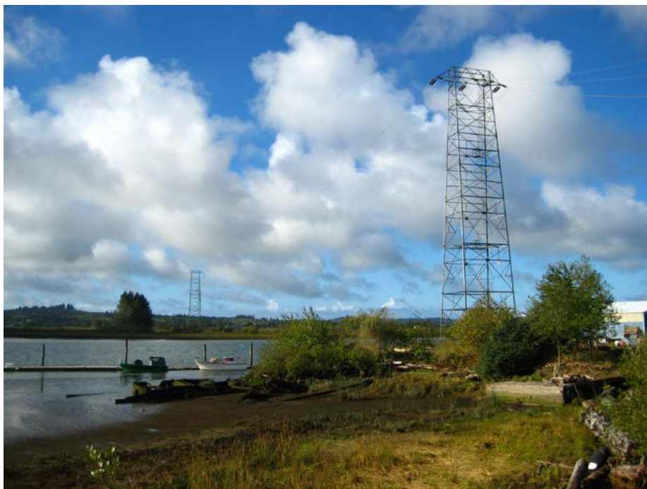
230-kv crossing of Youngs River
