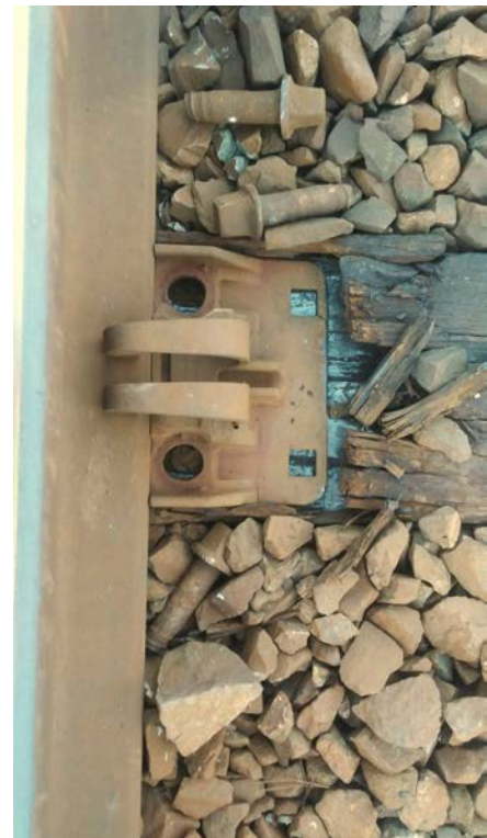
Image 1: Image of broken bolts that allowed rails to go wide, causing wide gauge.
